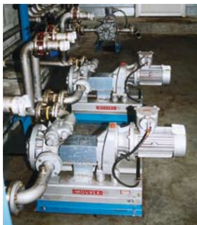
A-Series pumps, double bypass
