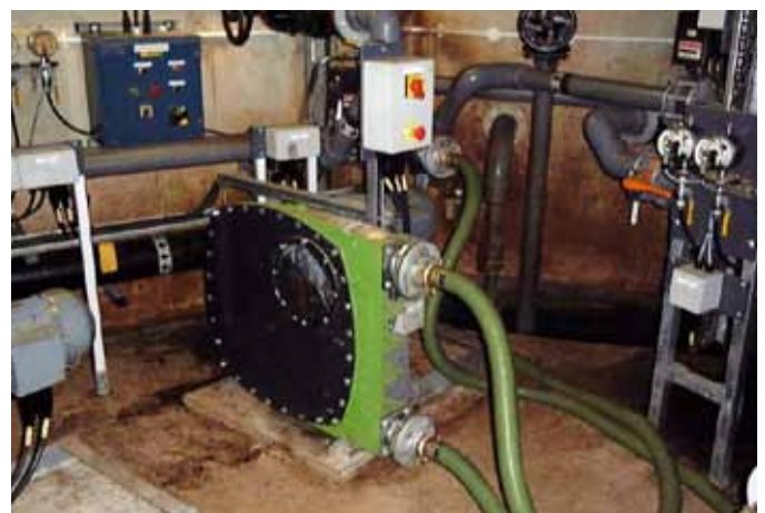
A Verderflex in a Ferric Sludge filter press application
