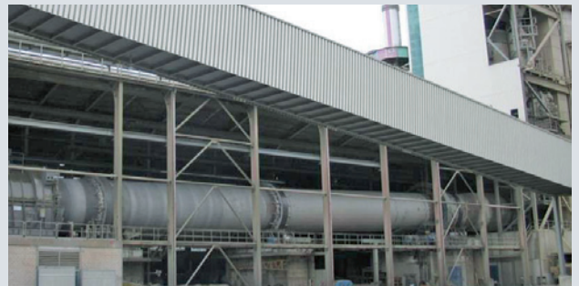
Cement industry – rotary kiln feed
