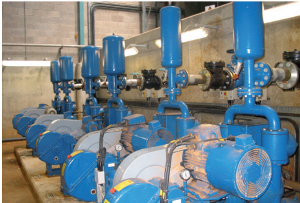
CM piston membrane pumps in a water treatment works in Northern Ireland
